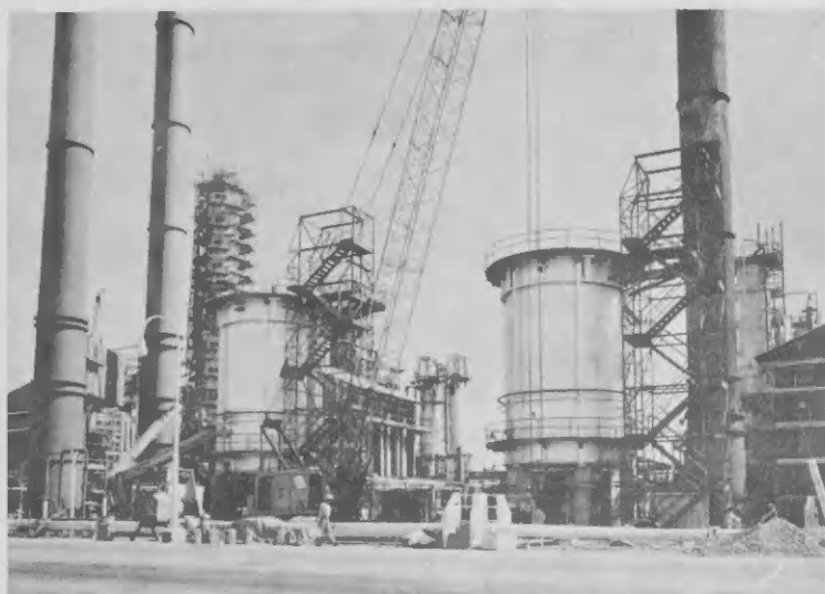
Construction on the modification to Nos. 9-10 Pipestills is taking shape, with most salient changes being the two cylindrical furnaces in foreground.
